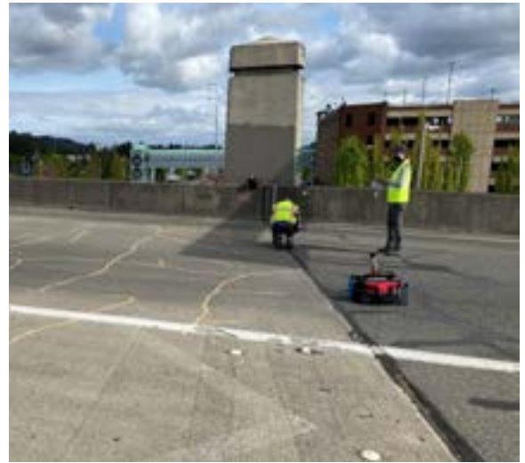
Photo A: 3rd Street SW Bridge - surface crack mapping
