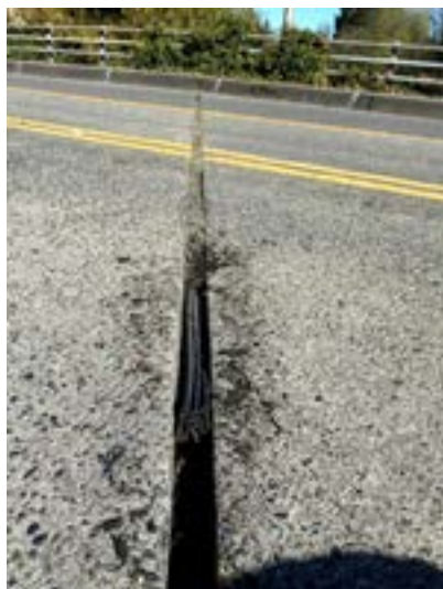
Photo B: Lea Hill Bridge expansion joint damage
